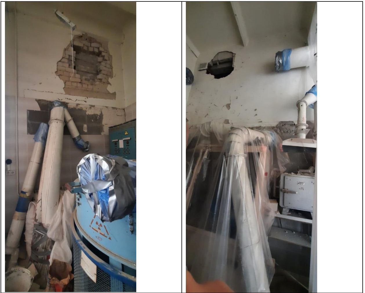
Fig. 2 – The destroyed technological equipment: muffle furnace, drying box, spheroidizer
